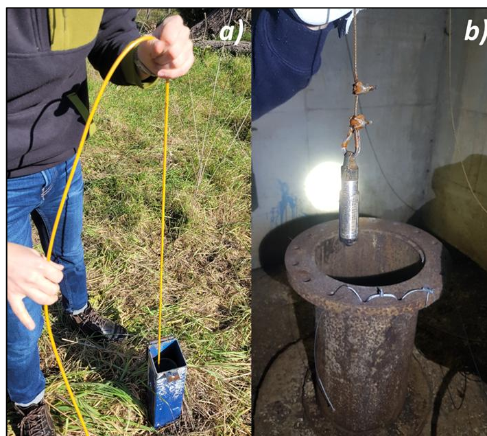
Figure 4.3. Diver sensors installation in (a) Benevento plain and (b) Dragone plain piezometers.
