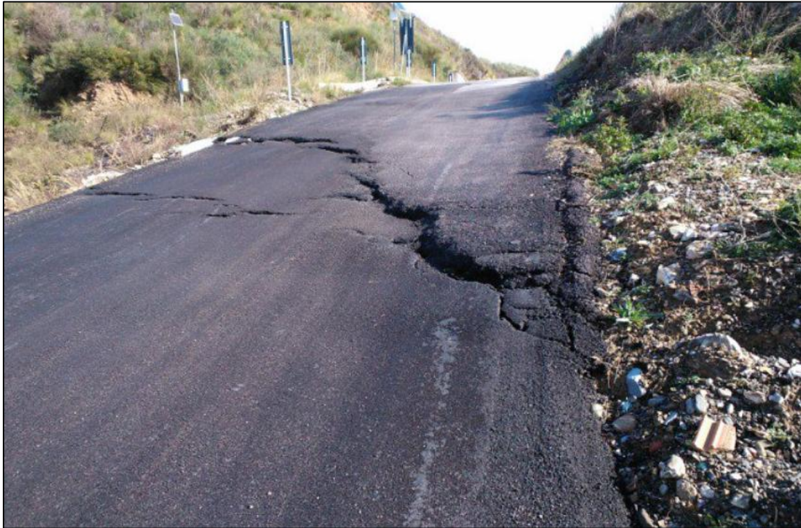
Figure 1.3 - Details of the damage on the provincial road ex SS447
