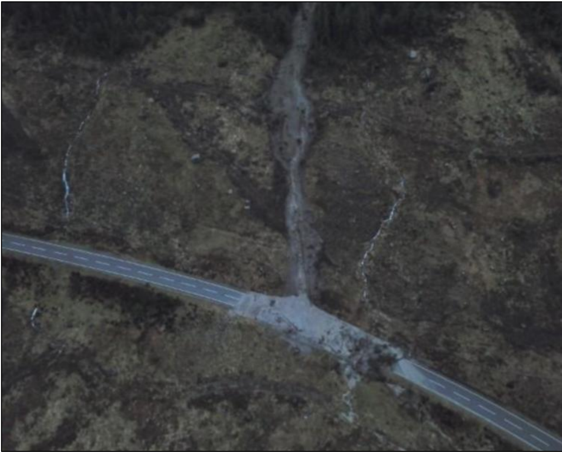
Figure 1.5 - Source: Helensburgh (2016). Landslide on route A83.
