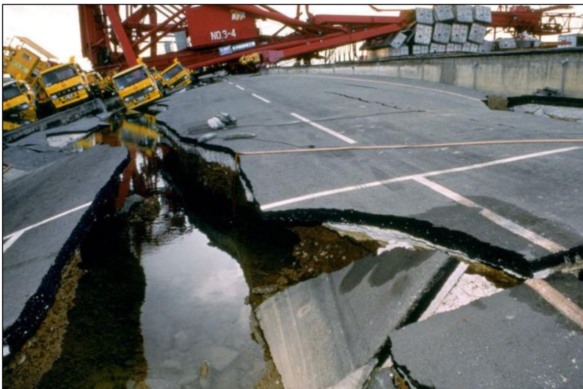
Figure 1.4 - The landslide affected the bridge.
