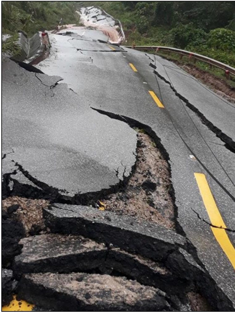
Figure 1.6 - Landslide damage caused to a road in Vietnam.
