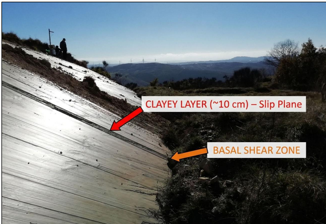
Figure 6.2 - Detail of the basal shear zone and slip plane. The field observation highlights a thin clayey layer (approximately 10 cm thick) acting as the main slip surface. The basal shear zone marks the mechanical discontinuity between the stable substrate and the overlying landslide material.
